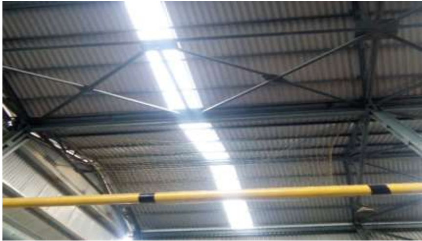
Daylight utilization using transparent Roof sheets
